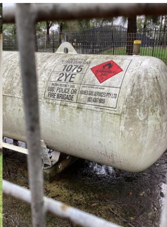
Photo 28: Photograph of above-ground tank, photograph taken facing north (taken 05/07/2022).
