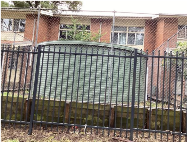
Photo 25: Example of rainwater tanks observed onsite, photograph taken facing north (taken 05/07/2022).
