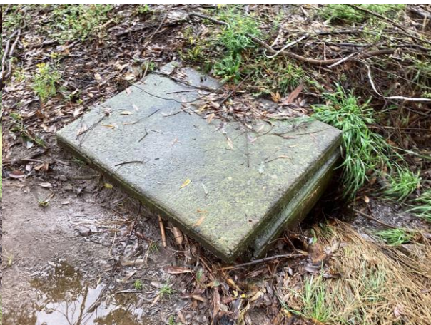
Photo 16: Example of stormwater pit located along the east perimeter of the field, (taken 05/07/2022).
